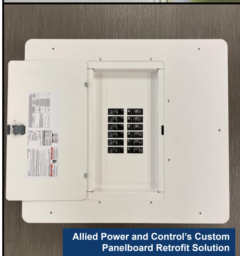
Existing facility distribution panel condition
